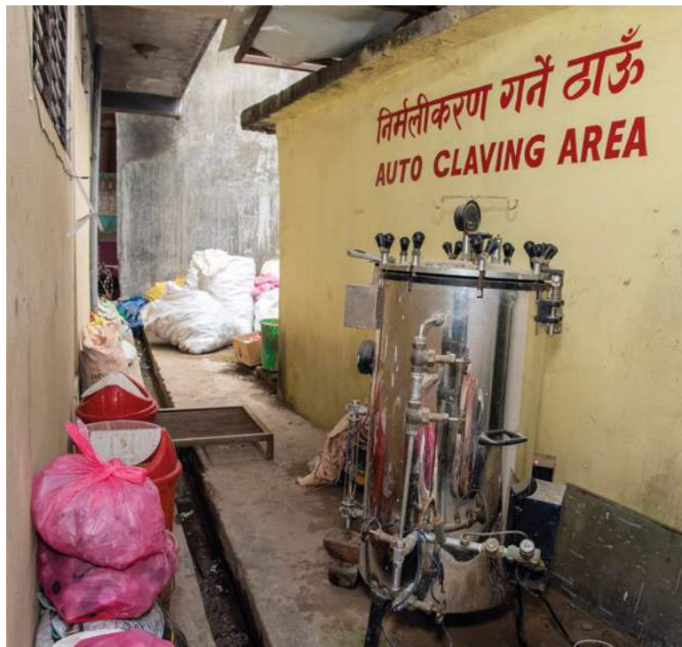
→ Hazardous healthcare waste from across the municipality is treated at the Primary Health Center.
